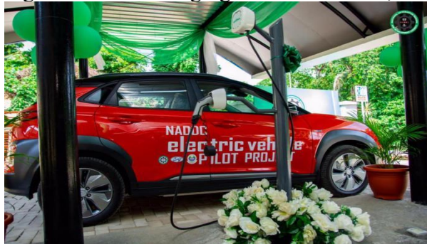
Figure 6.3: EV Charging station at Uni-Lag, Lagos.
