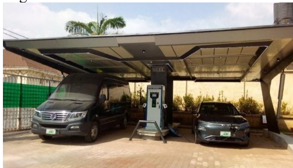
Figure 6.4: EV Charging station at NADDC Office, FCT, Abuja
