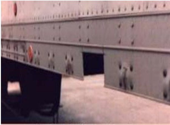
Fig 8 Truck Trailer Frame Corrosion
